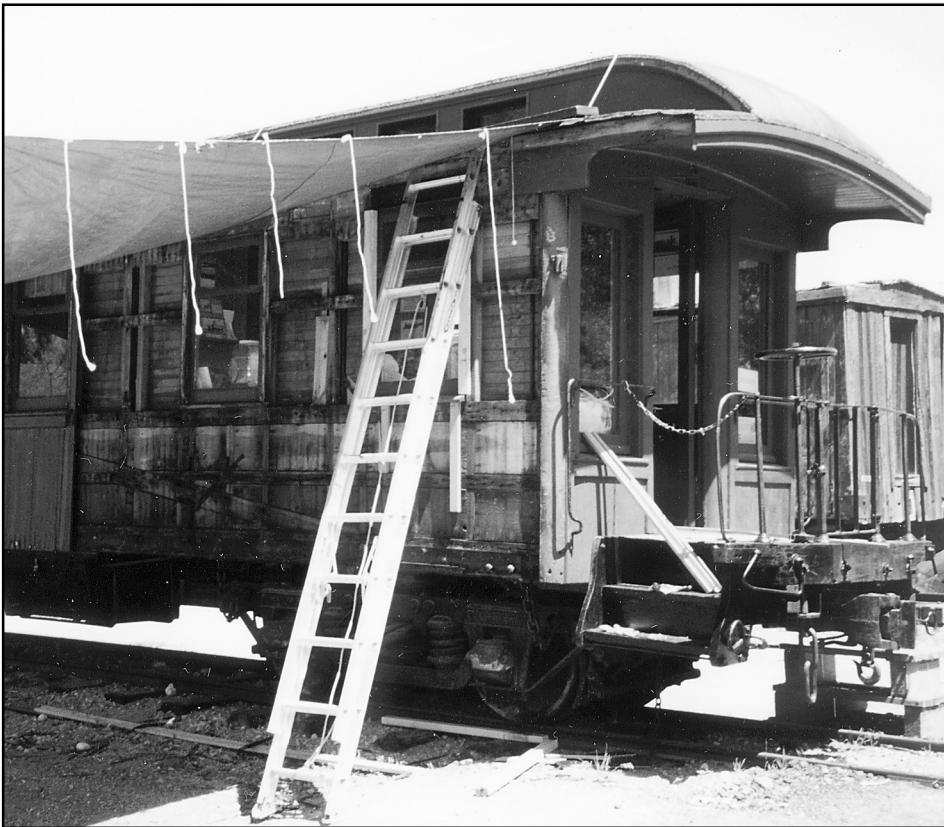
The area where the siding has been removed from the RICO is protected by a tarp. The side framing is in remarkably good condition considering that it is over 100 years old. – Photo © Bob Tully.
