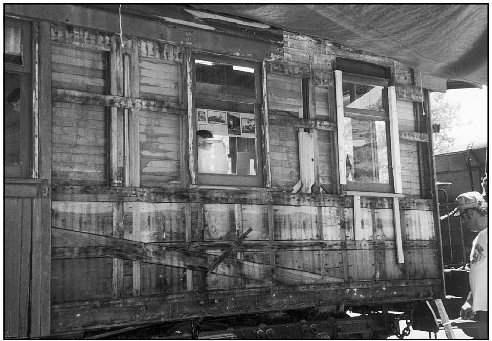
Denny Haefele measures wood pieces to replace the window frame on the north side of the RICO. – Photo © Bob Tully.
