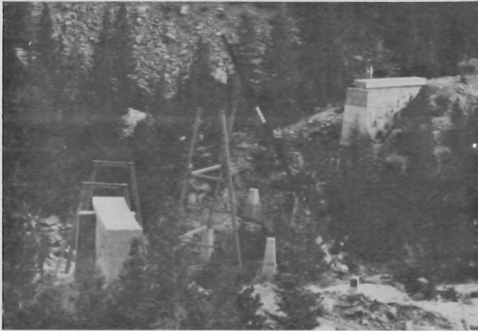
Overview of the new bridge with towers being raised to their positions on pilings. August 25, 1983.
